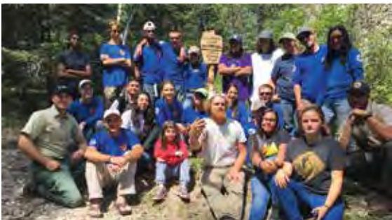
First Wilderness boundary signs installed for the Columbine-Hondo Wilderness with youth from stewardship organizations across the U.S. Photo: Rhett Spencer
